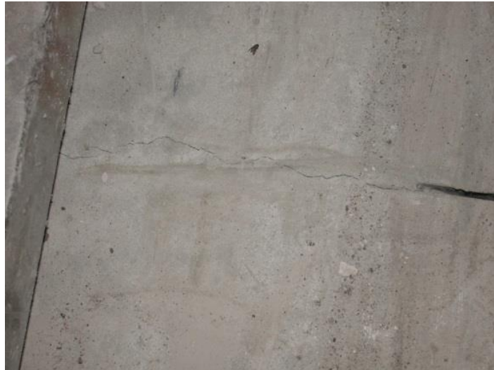
Figure 5-9: Cracking in the extension of the sawn shrinkage joint to the wall.
