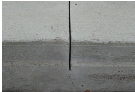
Figure 5-6: The crack under the sawn shrinkage joint shows the joint's mobility.
