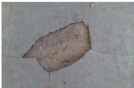
Figure 1-1: Delamination of a concrete floor.
