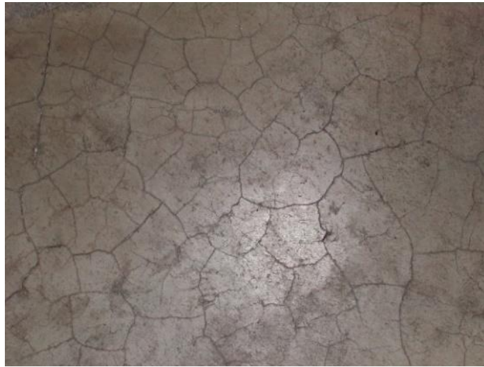
Figure 5-4: Microcracks (crazing) at the concrete surface due to differential shrinkage.
