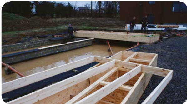
Construction of a wooden floor above a crawl space that does not comply with the recommendations from TIN 291.
