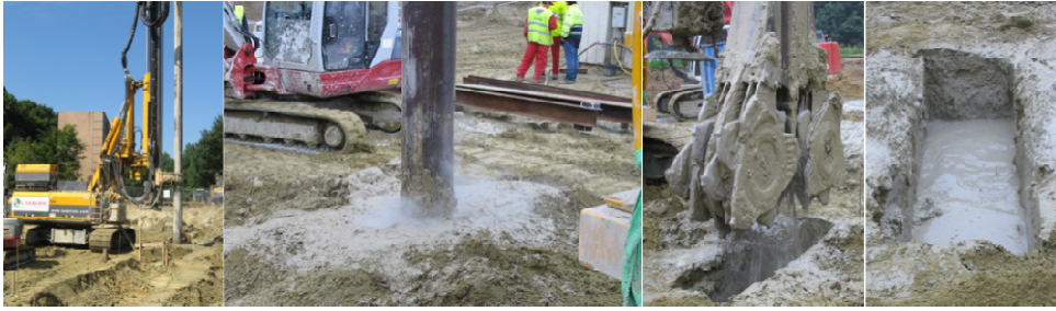
FIG. 1. Execution of a soil mix panel (type CSM) on the construction site of Heverlee (Belgium)
