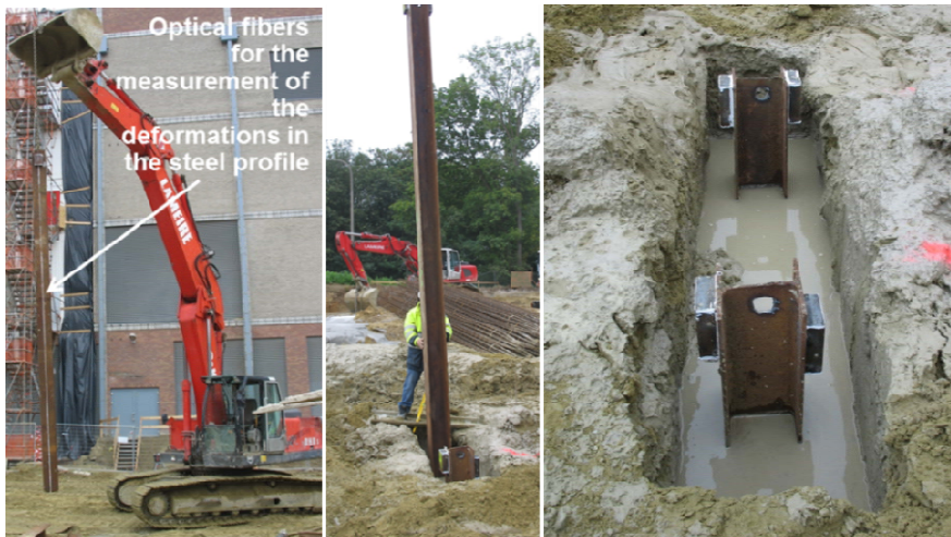
FIG. 2. Installation of an equipped steel profile in the fresh soil mix panel just after execution
