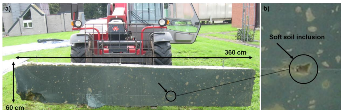
Figure 2: a) Saw-cut section of a CSM panel, b) enlargement of a soft soil inclusion
