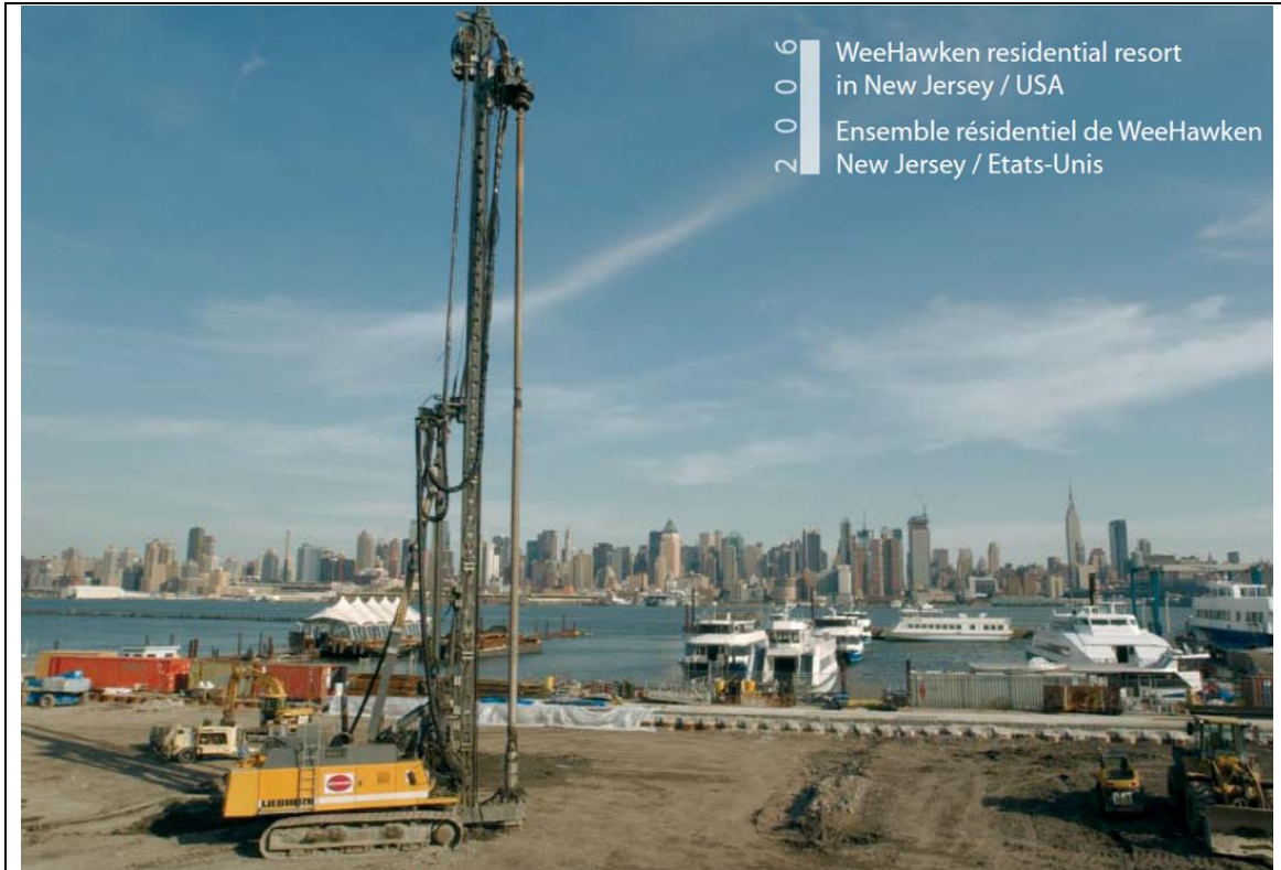
Figure 29: CMC installation on the construction site of the WeeHawken project in New Jersey, with the courtesy of Menard Company
