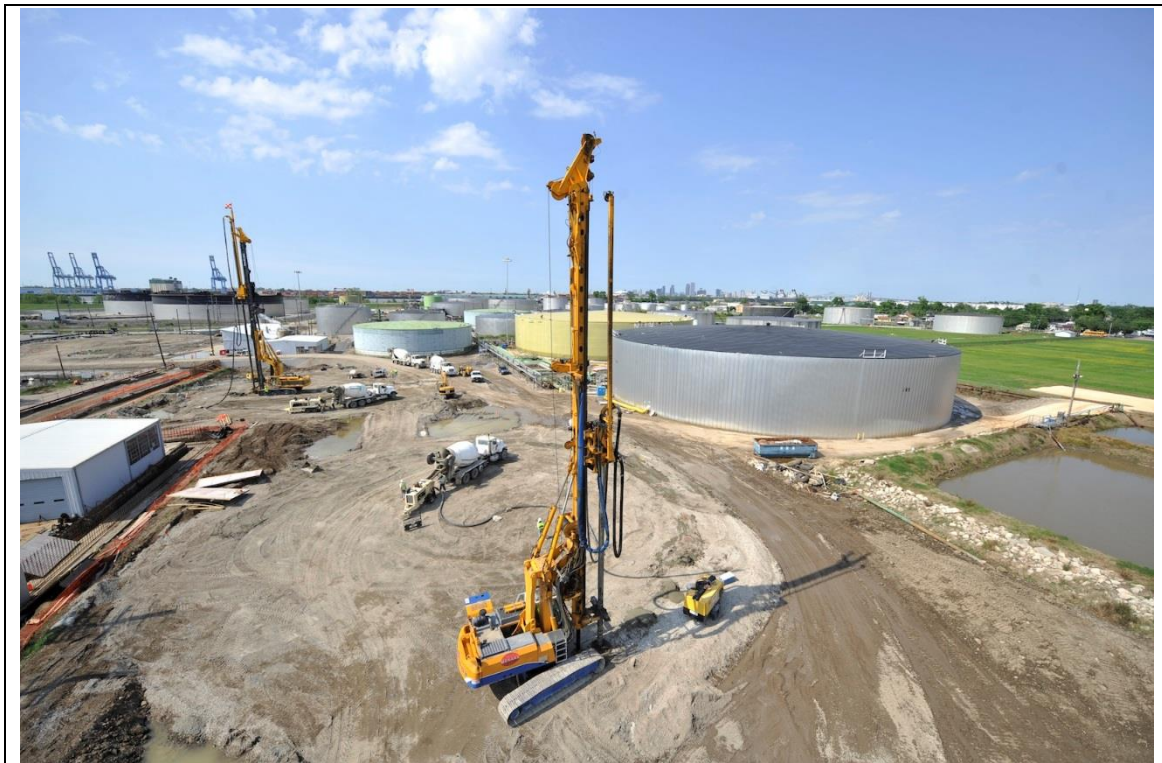
Figure 30: Installation of the CMCs on a construction site (oil terminal) located on the banks of the Mississippi River in New Orleans, USA
