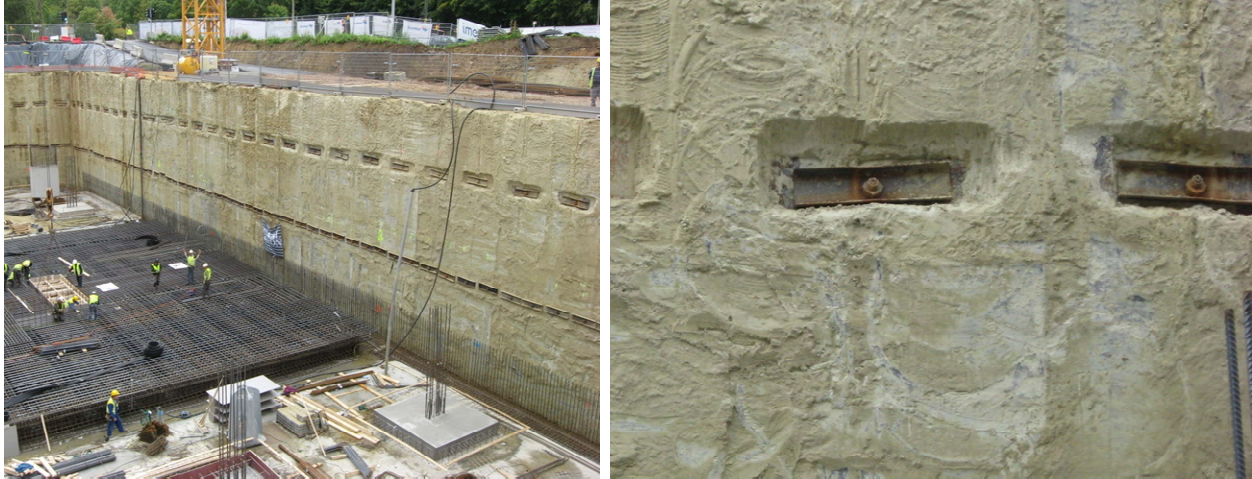
Fig. 1. Excavation realized with the help of an anchored CSM wall in Heverlee (Belgium)
