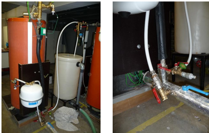
Figure 1 - Global views of the expansion vessel on the inlet connexion of the test tank.
