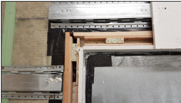
Figure 5. Vibrational decoupling of the reveals of the interior lining using resilient pads between timber laths.
