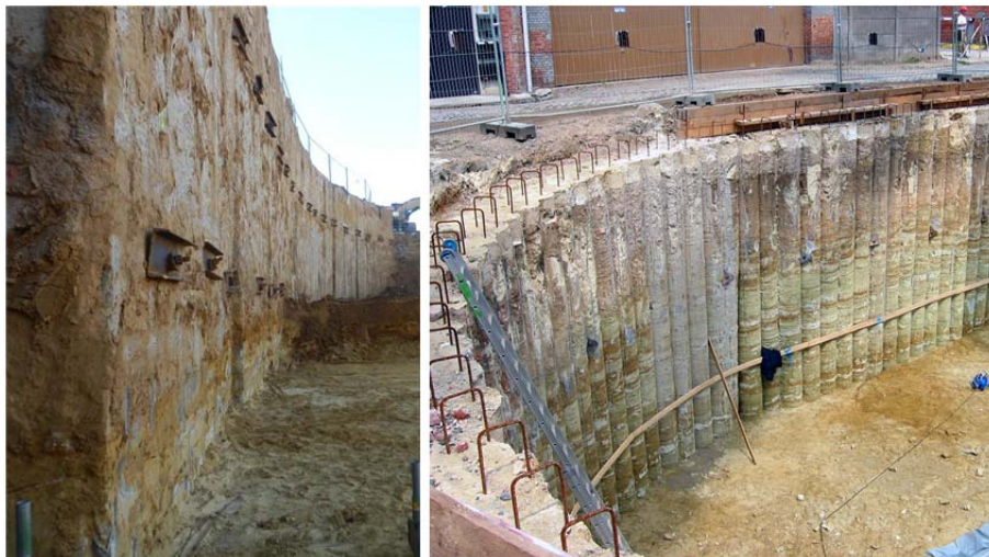
Figure 2. Soil mix retaining walls within the framework of excavation works in Belgium: soil mix walls built with CSM-panels (left) and with the C-mix shaft system of CVR nv (right).
