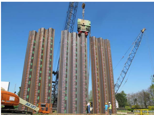
Figure 6. Vibrodriving of the last double sheet pile with the vibrator type Dieseko PVE 40VM on the site of the BBRI
