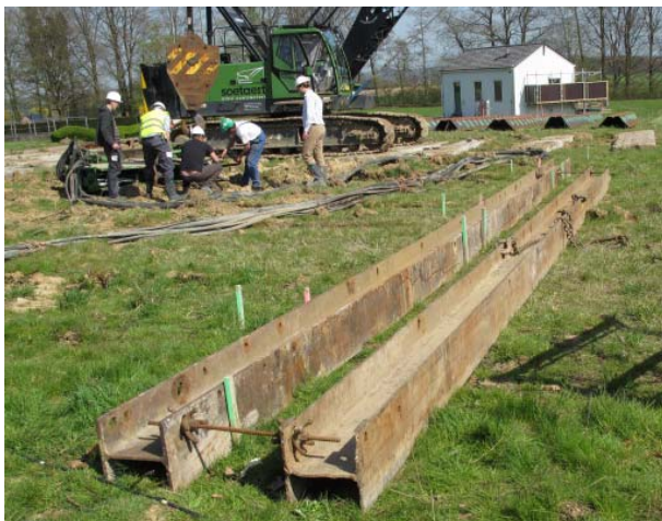
Figure 5. Steel guide used during the vibrodriving phase of the test campaign to guide the sheet piles into the ground
