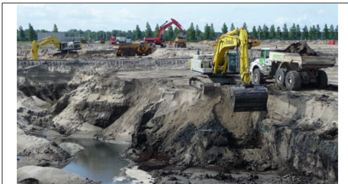
Photo 2: Photograph of the excavation of the compressible layers underneath the sand layer
