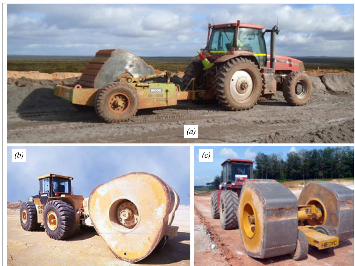
Photo 1: Rolling dynamic compaction modules: (a) 4-sided (Broons), (b) 3-sided (Landpac), (c) 5-sided (Infratech).
