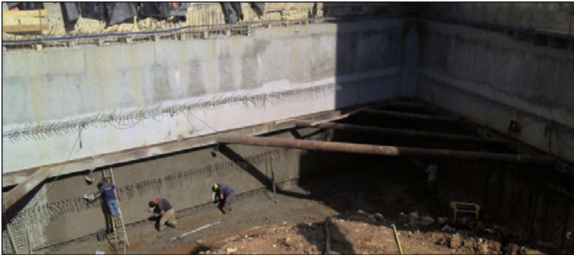
Figure 8: Partial view of the retaining wall with the steel waler beams, the internal struts and the concrete wall.
