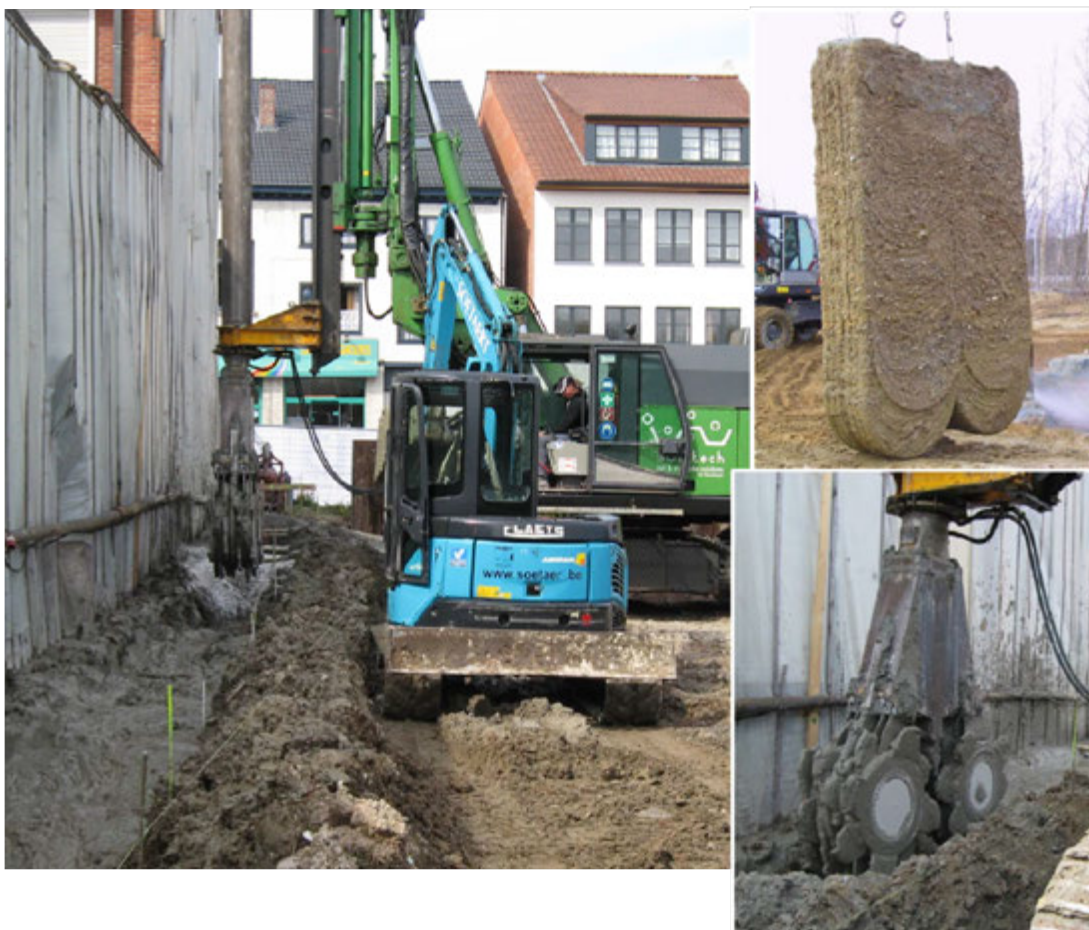
Figure 6: The cutting wheels of the CSM machine and the resulting CSM panel (Soetaert - Soiltech)
