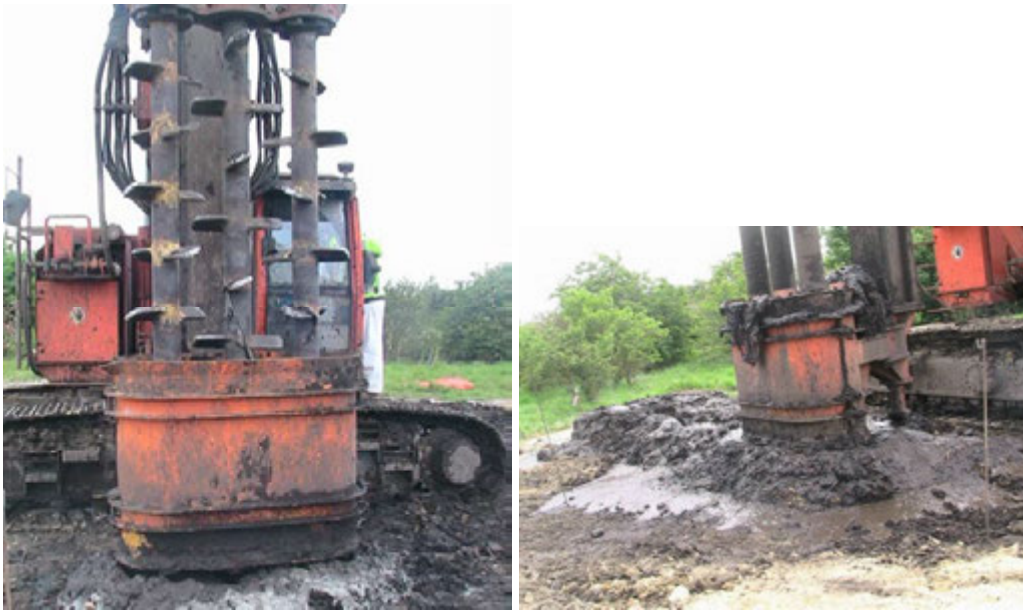
Figure 1: The triple auger system used in the field trials to install the PRB walls, low permeability wall sections and individual S/S sections
