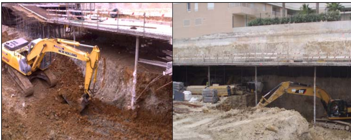
Figure 10: Views of the work during the execution of the second level of excavation.
