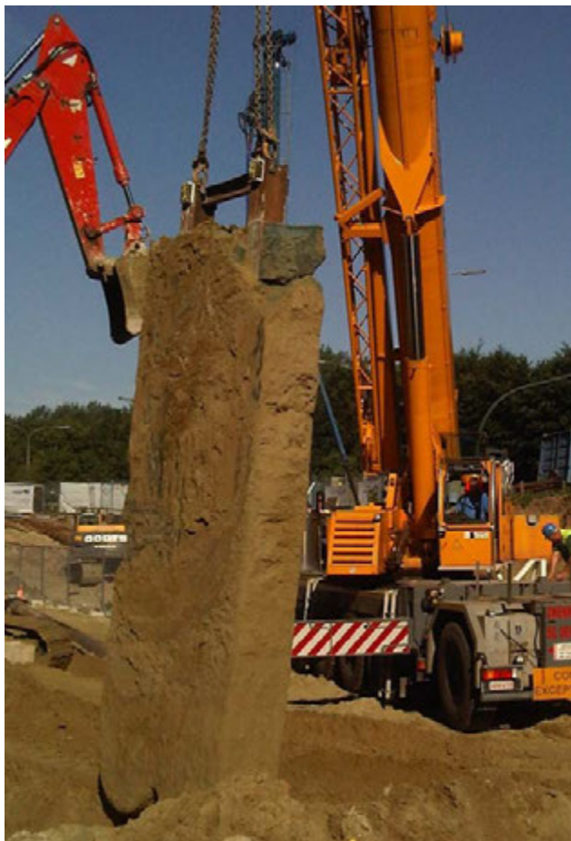
Figure 3: Excavation of an in situ executed CSM panel (Lameire Funderingstechnieken n. v.)
