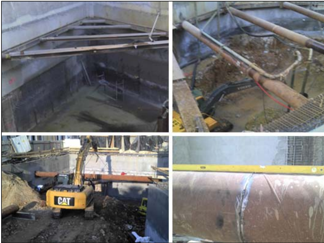
Figure 14: Different views of the work and a detail of a pipe strut.
