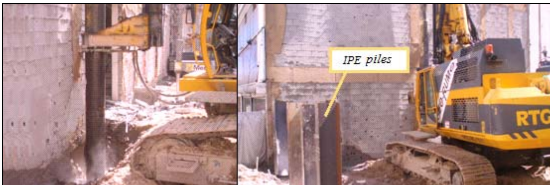
Figure 10: View of the execution of a CSM panel (on the left) and installation of the IPE piles (on the right).
