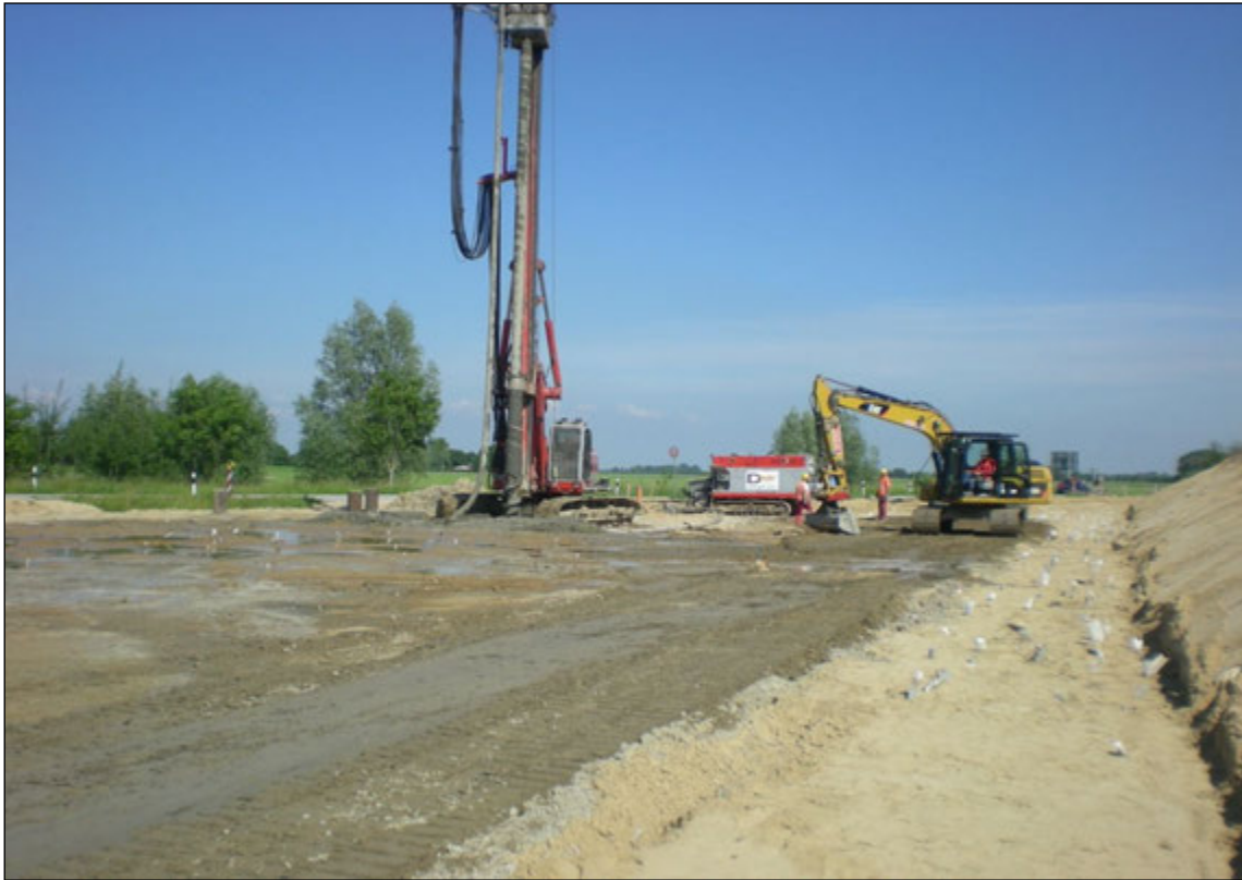
Photo 2: installation of CMC combined with vertical drains with water on the platform
