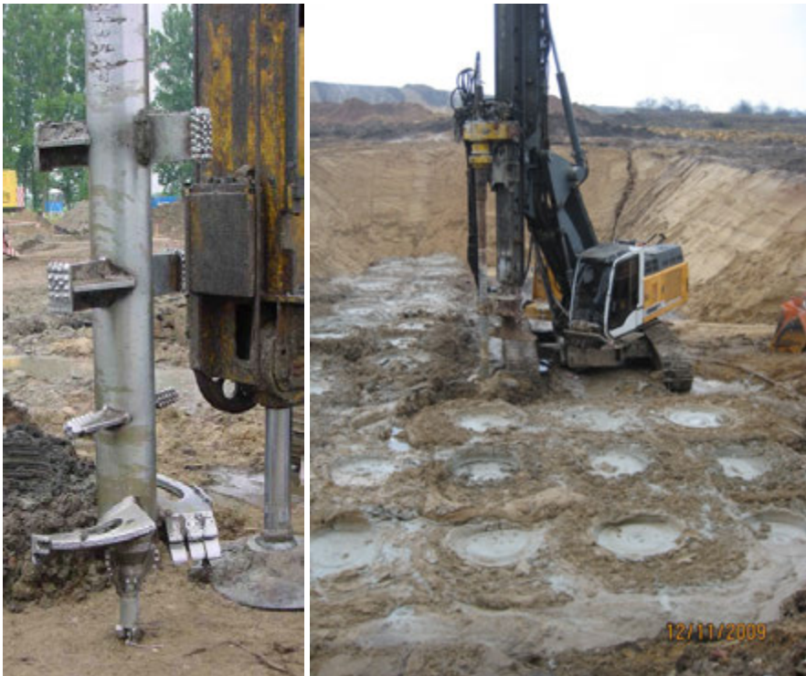
Photo 2: DSM Mixing tool with one shaft and four blades (left) and rig with single shaft mixing tool (right) (property of Keller Grundbau GmbH)
