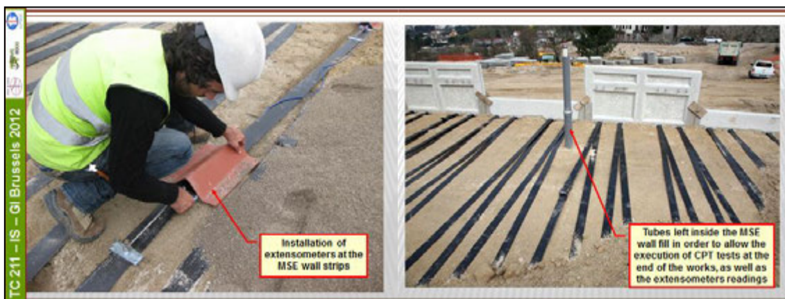
Figure 30: Devices adopted for monitoring the “Marão” Motorway M4B wall.
