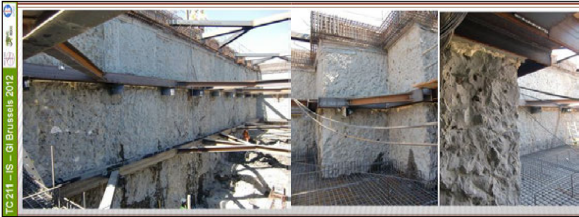
Figure 19: Views of the excavation works, with no water inflow, and details of the compatibility of the CSM panels with the internal structures.
