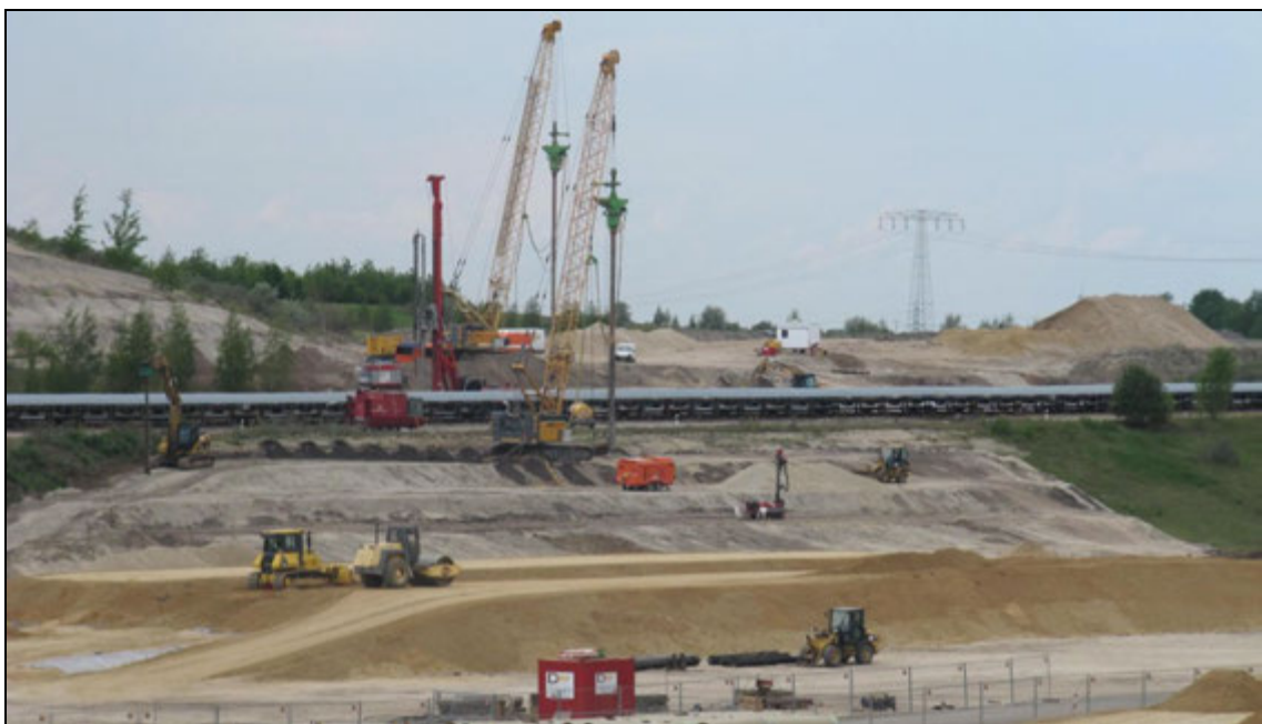
Photo 5 : Ripping holes for the two devices RSV, CMC directly on BW2 and PMT in front
