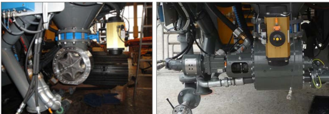
Photo 1: Star feeder with butterfly valve and silo; Photo 2: Rotary valve with hydraulic motor, gear box and coupling
