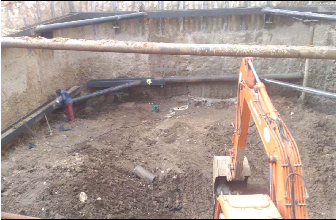
Figure 12: View of the work after the execution of the second level of struts.
