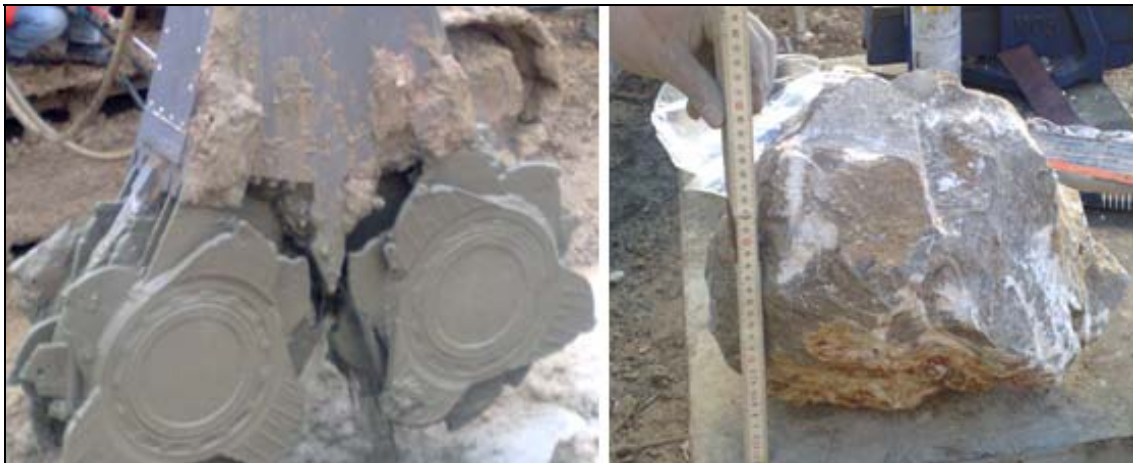
Figure 15: Cutting head used to the execution of the CSM panels (on the left) and example of a rocky block collected during the excavation (on the right).
