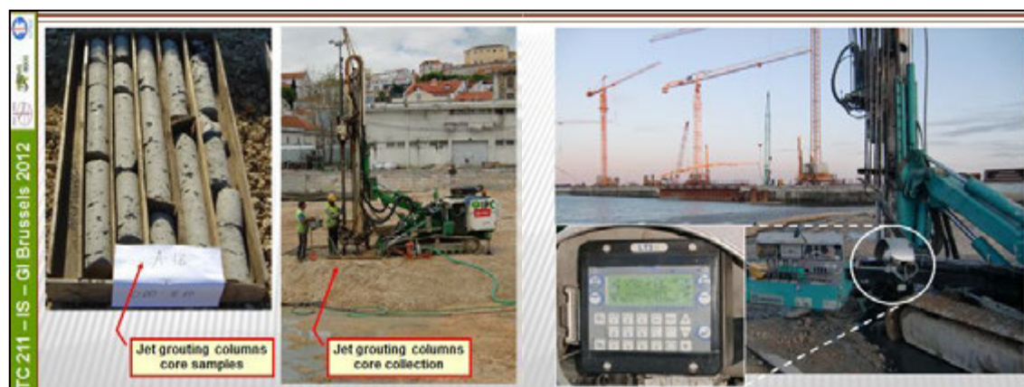
Figure 10: Quality control and quality assurance of the jet grouting columns: core samples and parameters registration (LT3).
