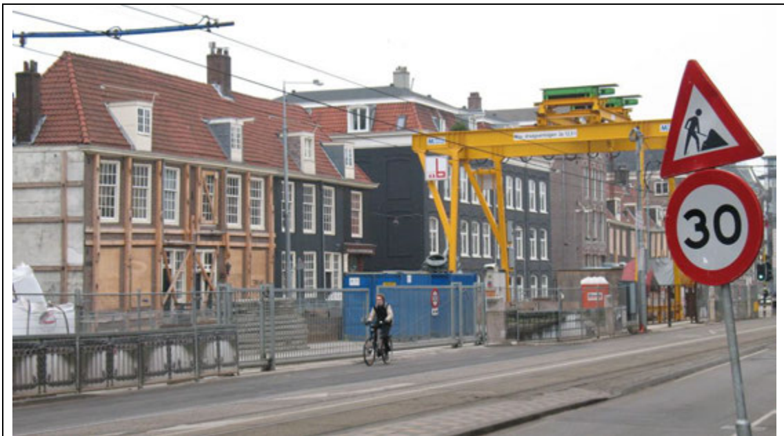
Photo 1: Damaged historic houses adjacent to Vijzelgracht Station
