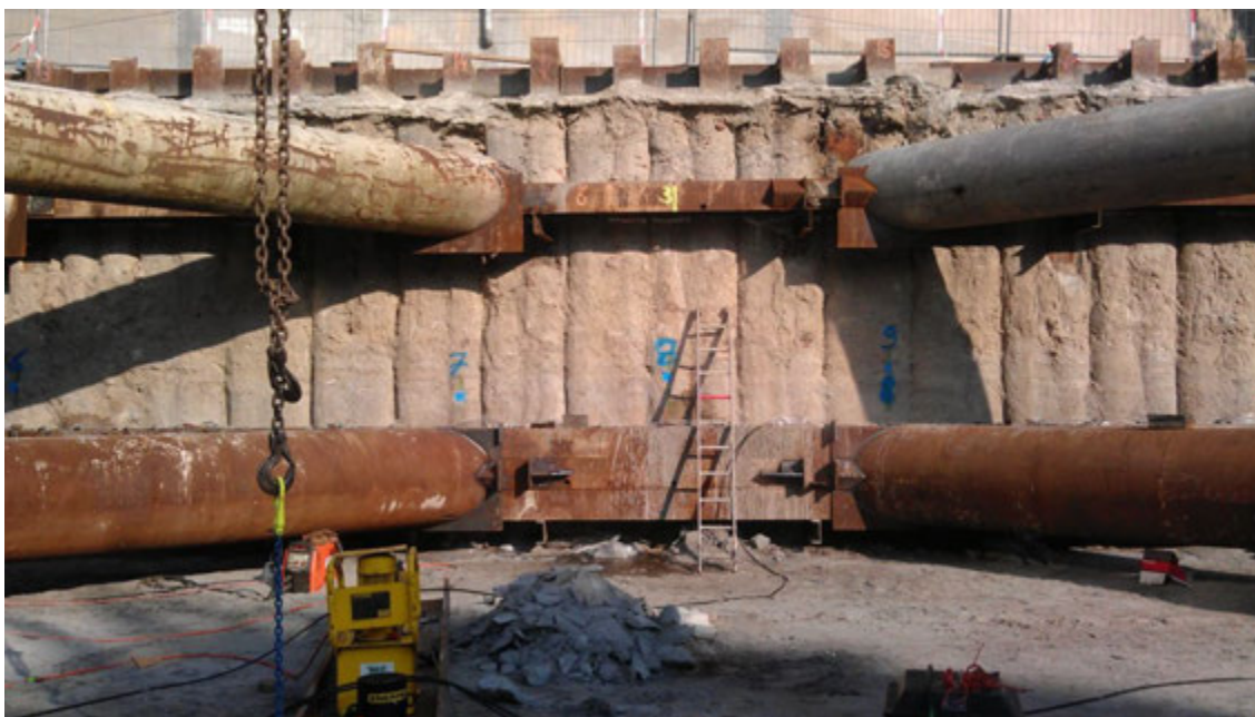
Figure 9b: Frontal view of excavation level -1 with struts, piles wall and bottom part of the Rotonde
