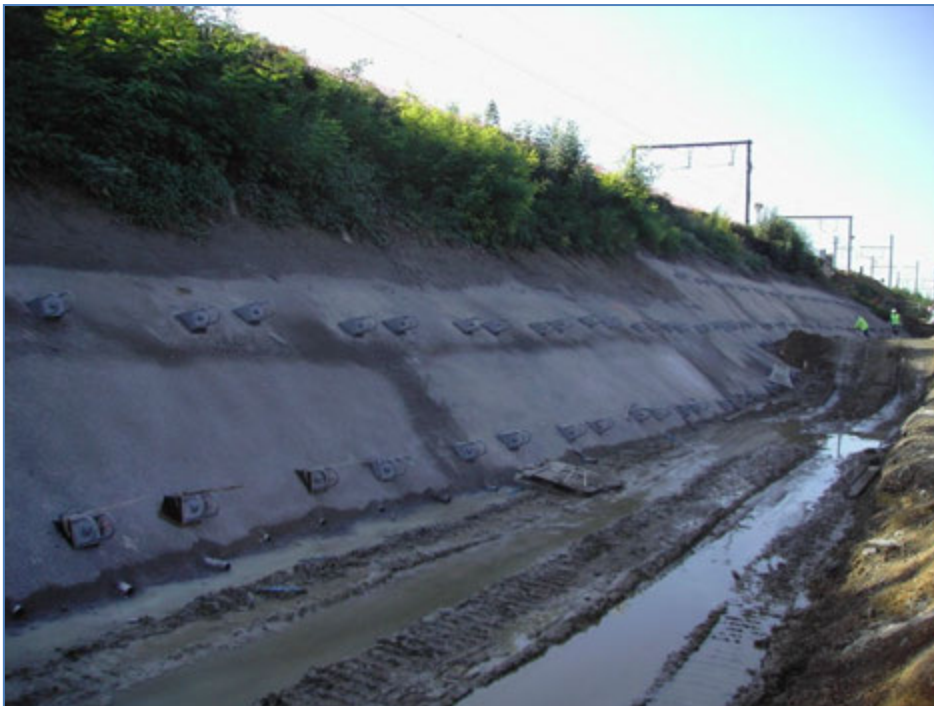
Photo 4: Soil nails with shotcrete and nail heads with rings to connect tube and geogrid
