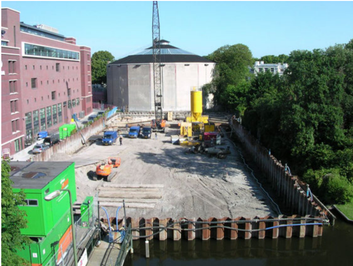
Figure 6: Overview of the site; left Hilton Hotel, middle PM & compensation grouting equipment
