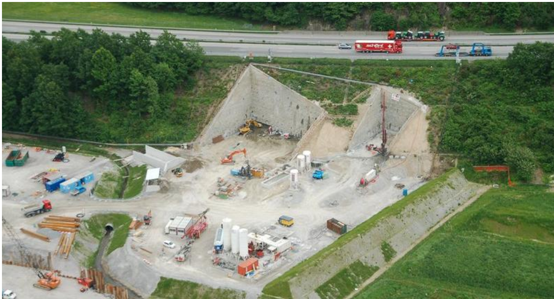
Figure 2: Aerial view of the north portal of the Tunnel during construction with the A2 motorway. Source: Alptransit SA Bellinzona
