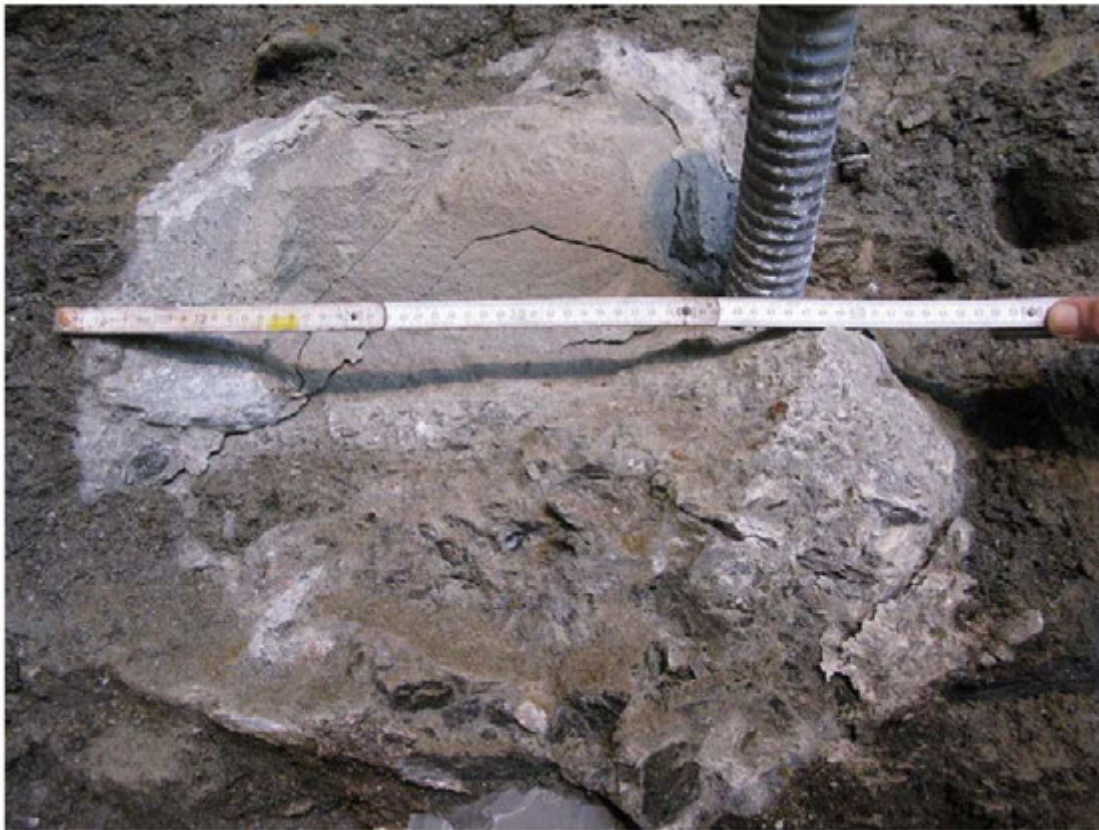
Figure 18: deviation of pile within jet grout column
