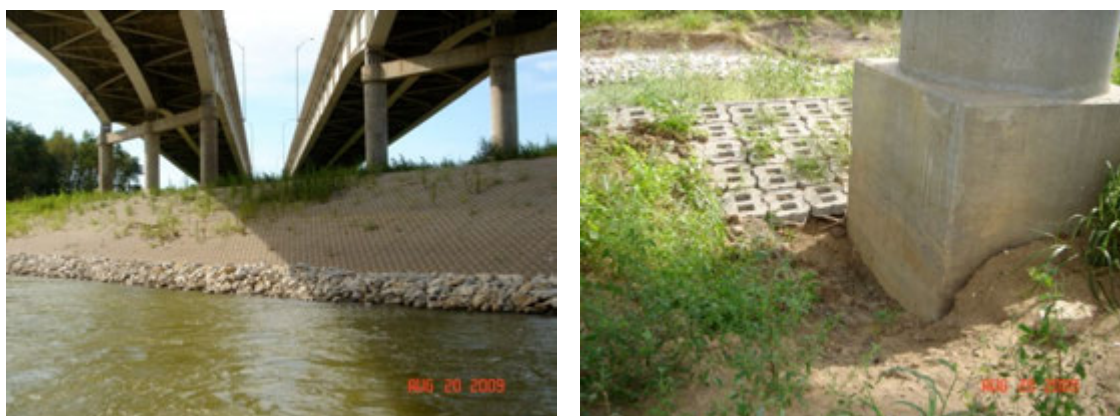
Figure 5: Interstate 35 bridge crossing the Trinity River south of downtown Dallas. The frame on the left is a view looking West. The frame on the right shows erosion under one of the piers of the East-bound lanes on the West bank piers and the Revetmat sloping at the top of the slope.
