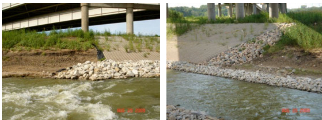
Figure 6: Left frame shows erosion downstream of the revetmat on the West bank. Right frame shows erosion and riprap placed on the upstream side of the West bank.
