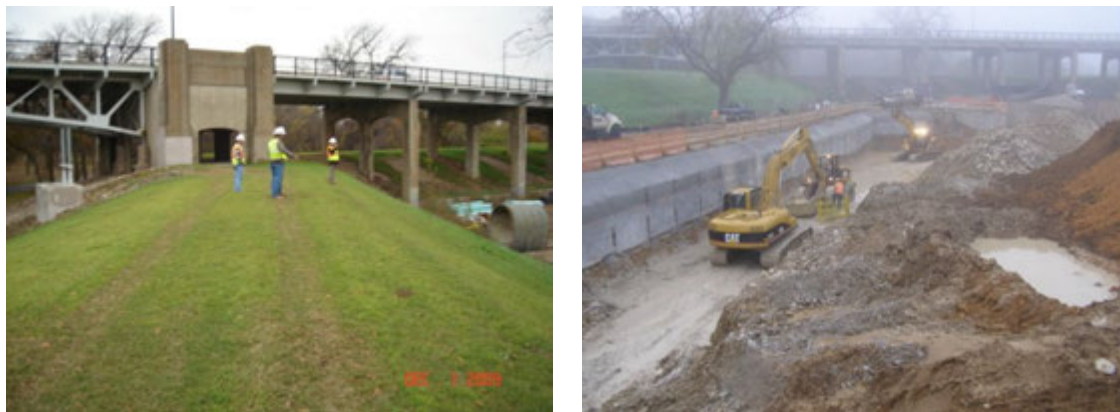
Figure 4: Lancaster Avenue Bridge in Fort Worth, Texas. The piles were installed in 1938 about 18 years after the levee was upgraded. Second frame shows excavation close to the levee in 2009.
