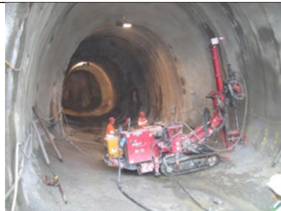
Figure 9: vertical jet grouting under the concrete beams in the first 9 meters of the tunnel
