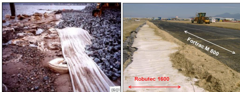
Figure 6: Example of horizontal geosynthetic reinforcement on top of already covered GECs for heavy loaded sensitive runways (left) and under a land reclamation embankment (GECs still visible) (right)
