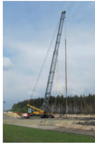
Wind Power to Lauzitsring GERMANY
