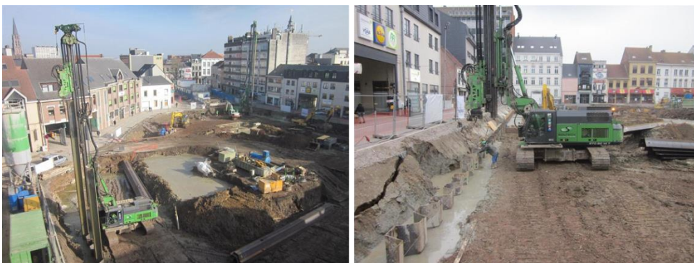
Figure 48: Installation of the sheet piles into the fresh soil mix material, after Leemans (2012)
