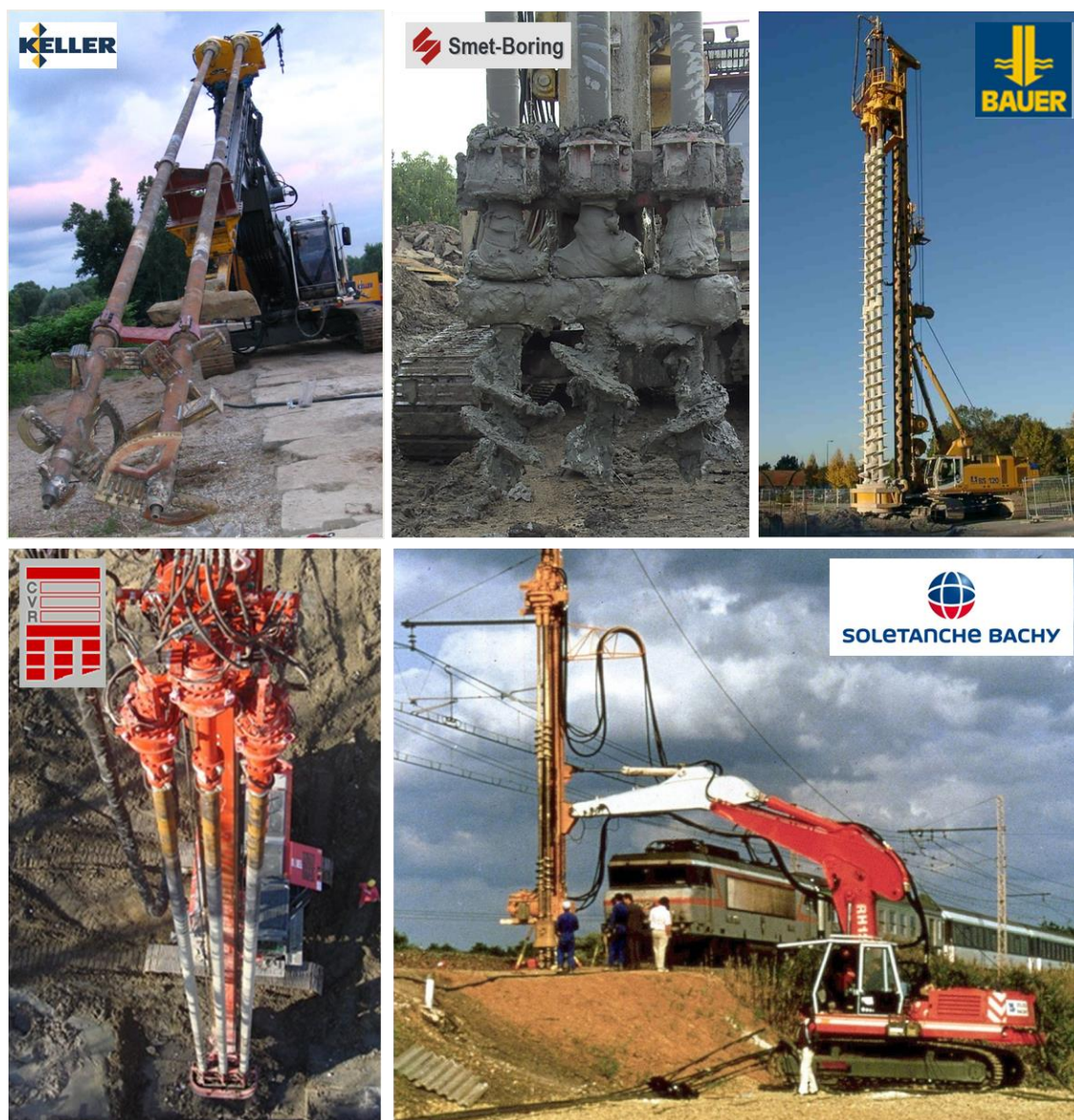
Figure 10: Wet mixing systems in double and triple shaft configurations, after Topolnicki (2012) , Denies (2012) and Borel (2012) with the courtesy of Keller, Smet-Boring nv, Bauer, CVR nv and Soletanche Bachy
