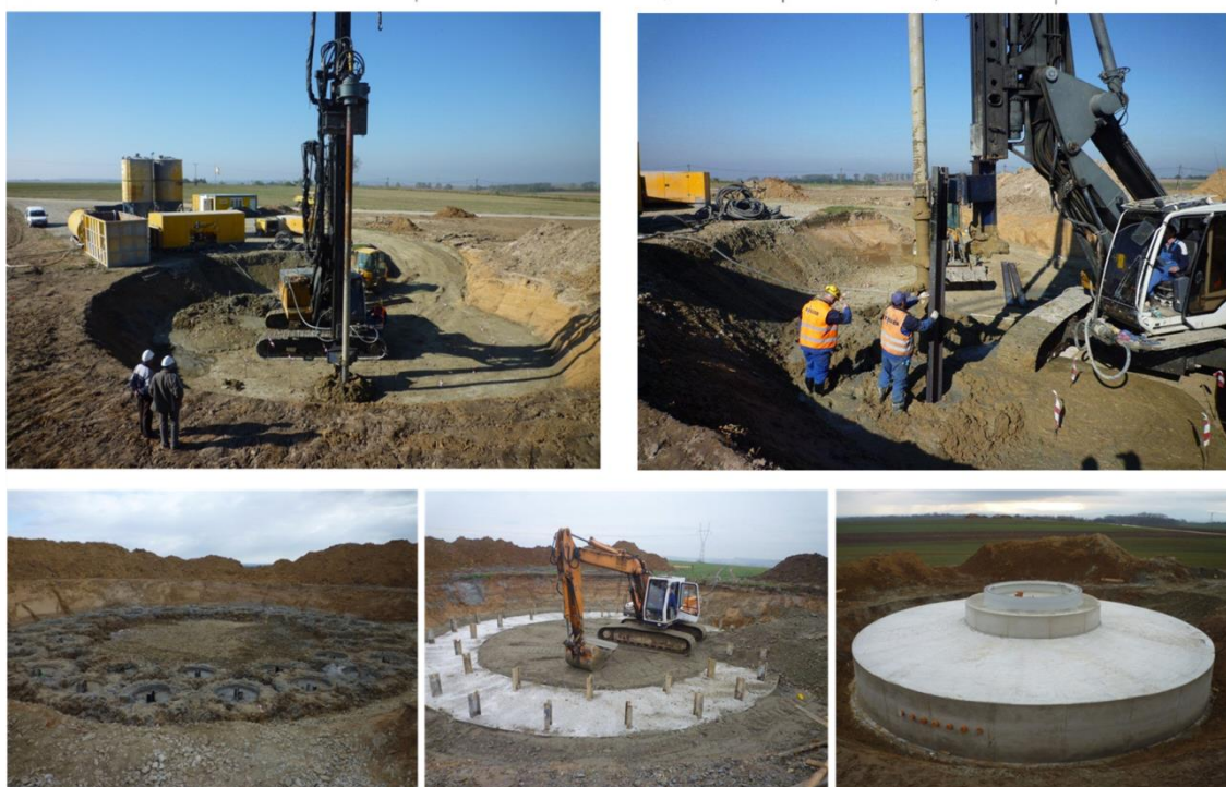
Figure 43: Examples of various structures supported by DSM elements – third part, after Topolnicki (2012)
