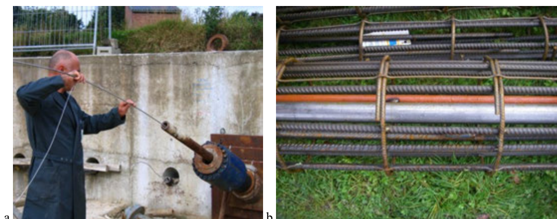
Figure 64: Examples of lost instrumentation systems integrated in a reservation tube after the installation of (a) an anchor and (b) a reinforced soil cement column, from Huybrechts (2012)
