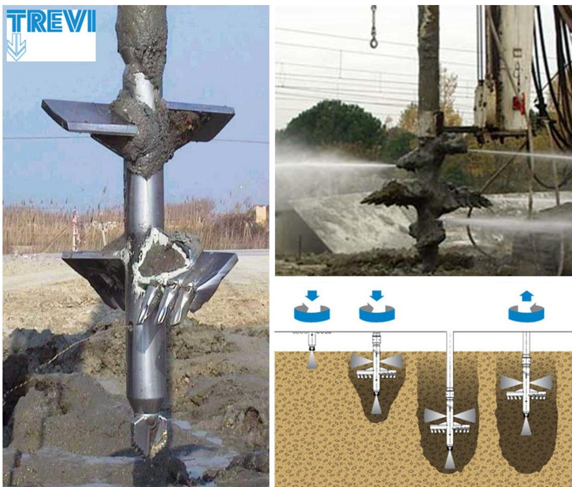
Figure 8: Trevi Turbojet technique (column diameter of 40 to 150 cm), after Topolnicki (2012) with the courtesy of Trevi
