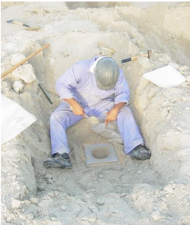
Figure 58: Technician performing in-situ density determination at 1 m deep excavation by applying the sand replacement method
