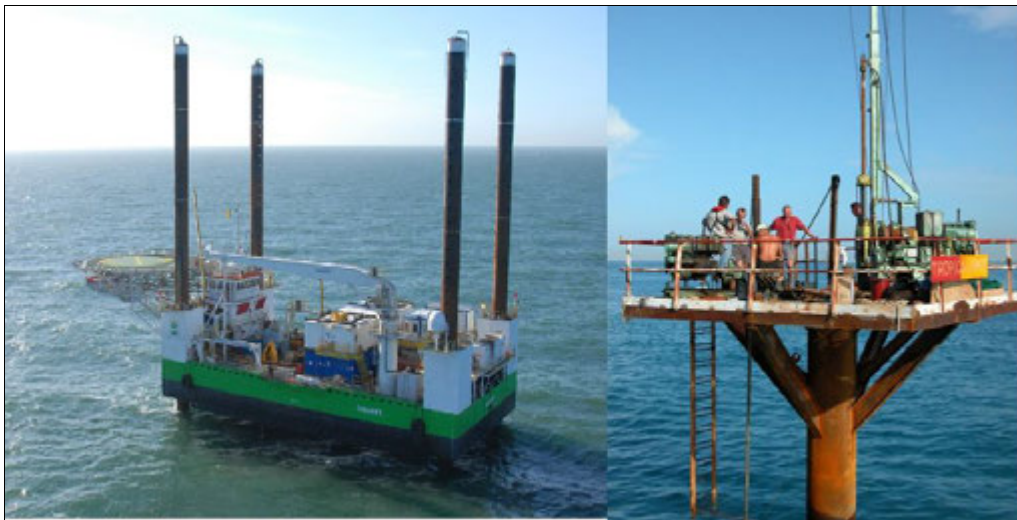
Figure 8: Stable working platforms for nearshore marine site investigations: jack-up platform Vagant (left) and monopole (right)
