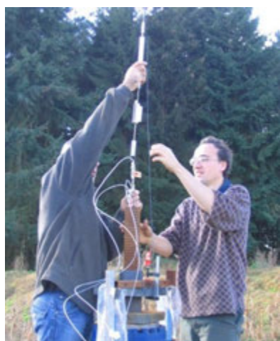
Figure 65: Installation of a retrievable instrumentation system in a reservation tube installed in a vertical anchor, from Huybrechts (2012)
