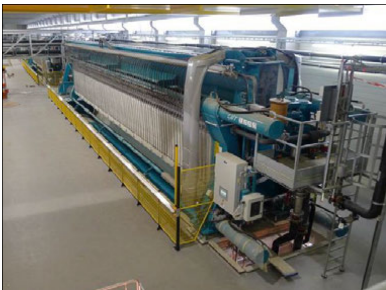
Figure 53: Mechanical dewatering by chamber filter presses at the Amoras project, Antwerp, Belgium
