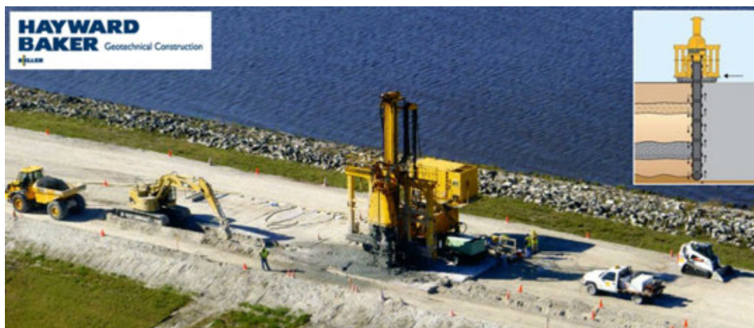
Figure 16: TRD soil mix walls with the courtesy of Hayward Baker and Keller
