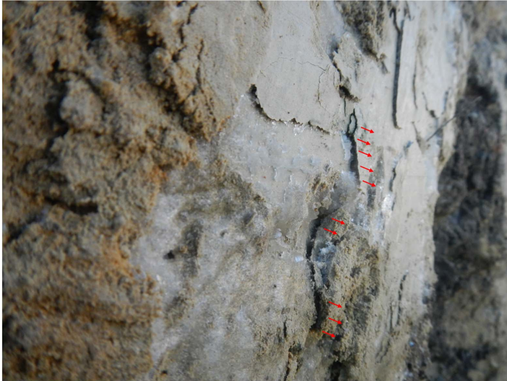
Fig. 3. Illustration of the “bursting”/shedding process resulting from the freeze-thaw cycles – side view – the picture is taken on November 30, 2016, a few days after execution of the column
