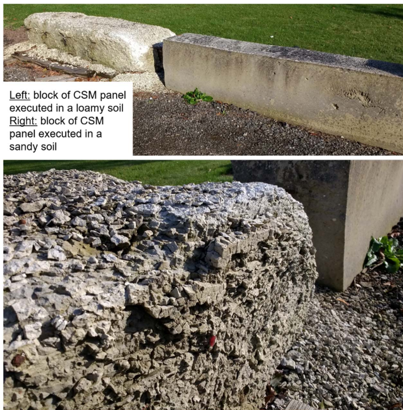
Fig. 4. Picture of two blocks cut in CSM panels excavated from two construction sites in Belgium - The picture is taken in October 2019, nine years after execution and excavation of the two panels
