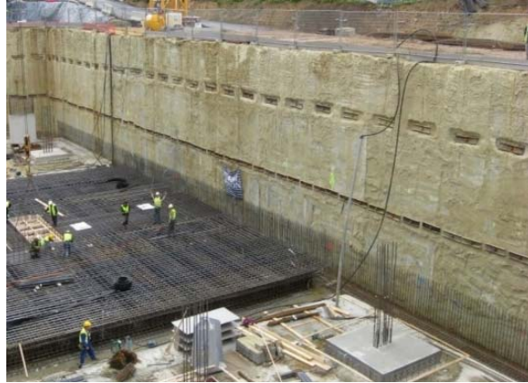
Fig. 1. Retaining wall made of secant reinforced CSM panels – construction site in Belgium
