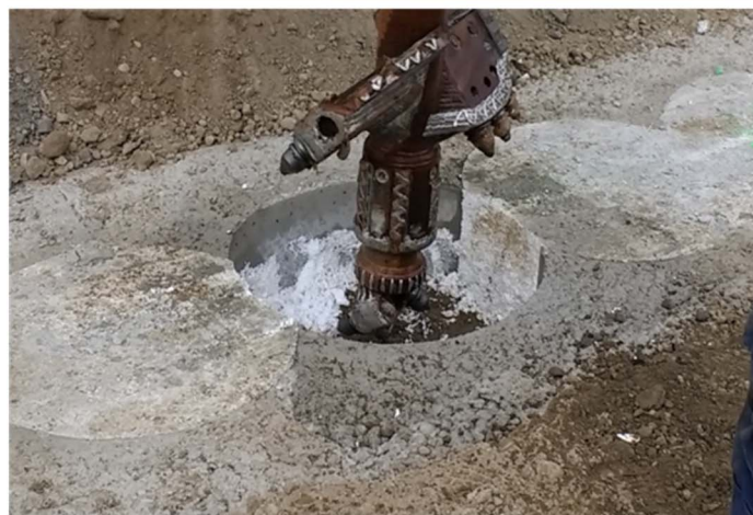
Fig. 21. Concrete beam with reservations (filled with expanded polystyrene) used to reach the execution tolerances for the alignment of the soil-cement columns
