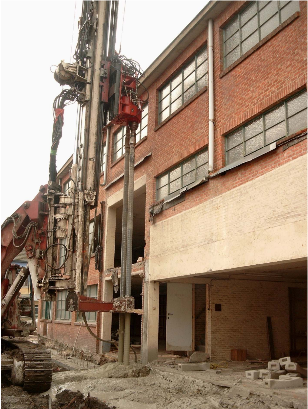
Fig. 12. Execution of secant soil-cement columns in double shaft configuration (with the courtesy of SMET F&C)
