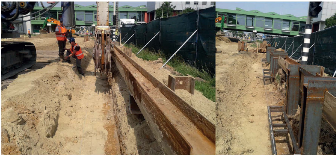
Fig. 20. Guide frames (left): used to reach the execution tolerances for the alignment of the soil mix panels executed along the horizontal steel beam; and (right): for the positioning of the steel beams in the soil mix material after extra steel frames are attached to the horizontal beam (Pictures with the courtesy of Hoffmann)
