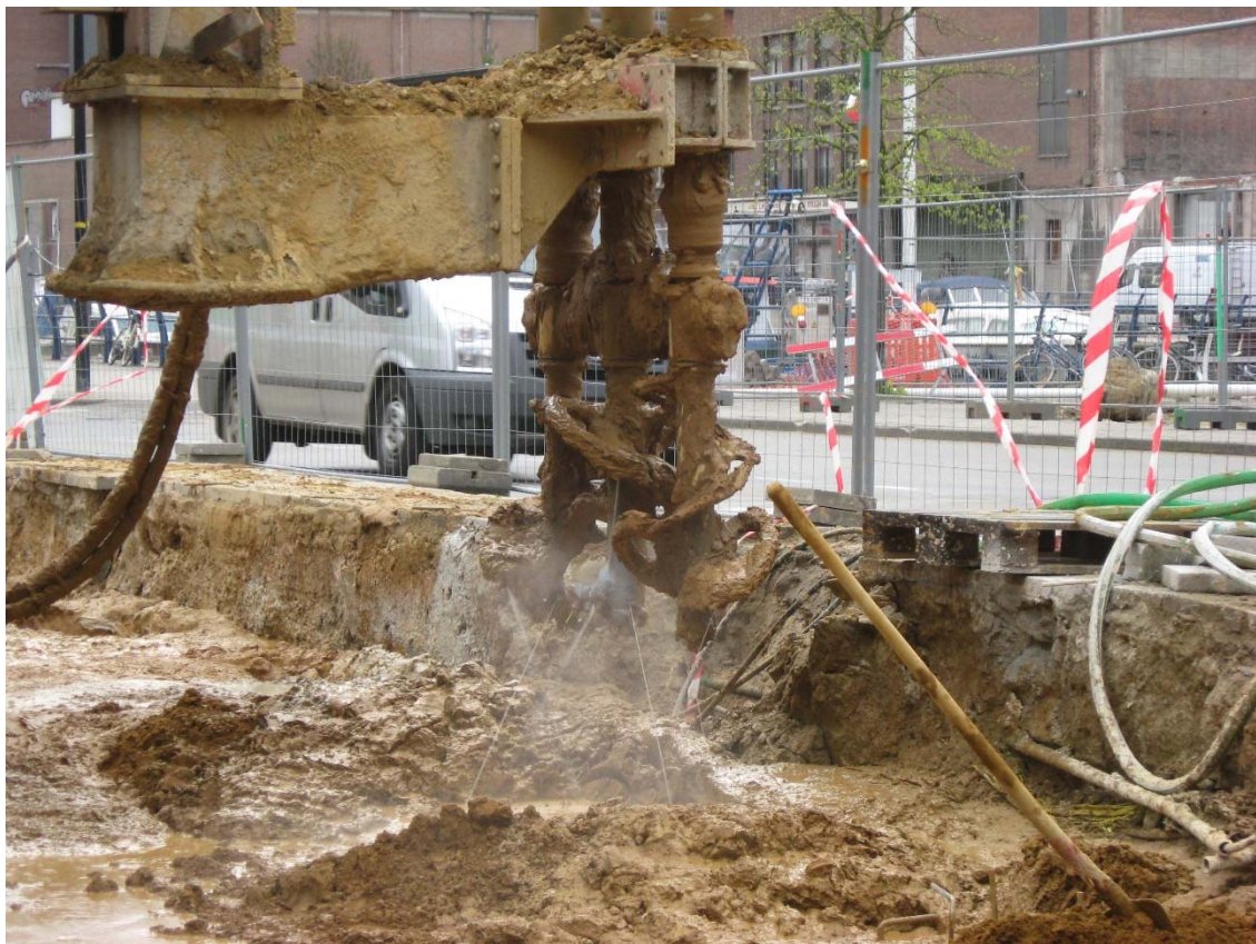
Fig. 13. Execution of secant soil-cement columns in triple shaft configuration (with the courtesy of SMET F&C)
