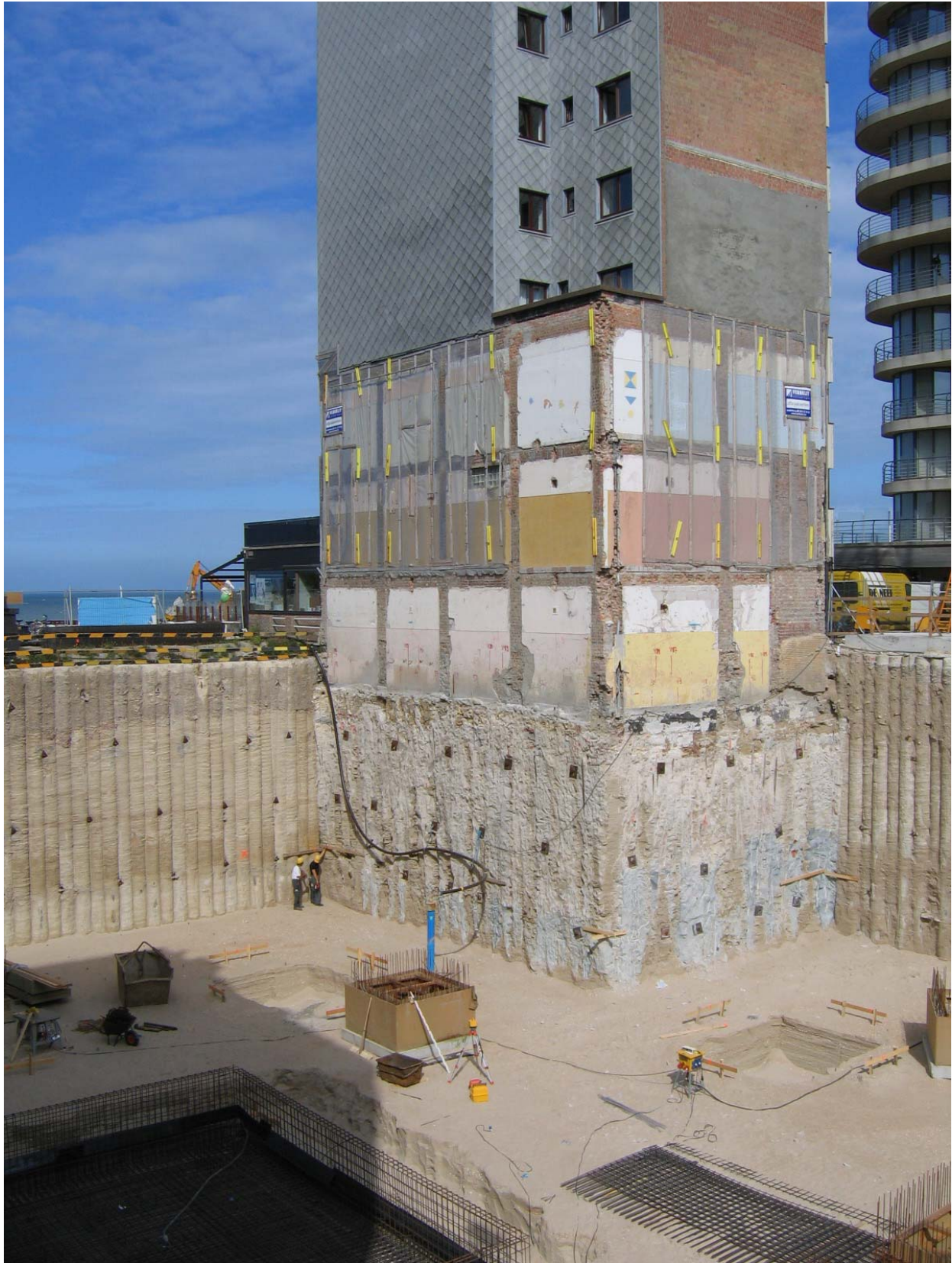
Fig. 5. Anchored soil mix wall (made with the TSM technique) used as retaining wall for the realization of an excavation and underpinning of an existing building (Smet F&C)
