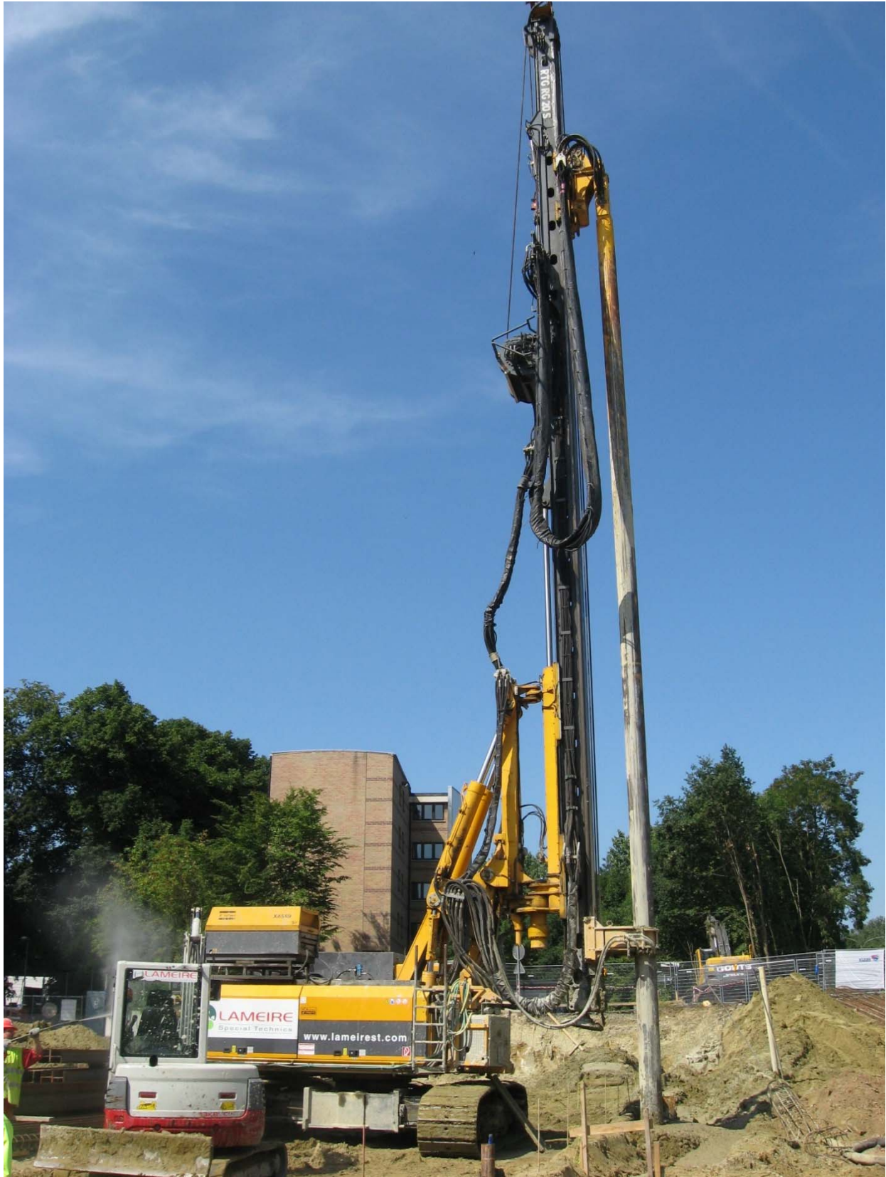
Fig. 14. Execution of a soil mix wall with secant panels performed with the CSM technique – the cutters are mounted on a cylindrical kelly (with the courtesy of Lameire funderingstechnieken nv)
