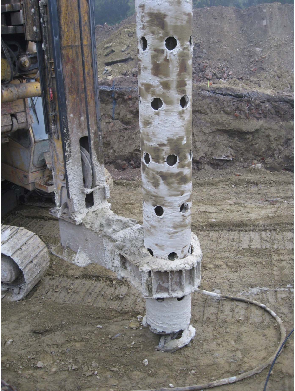
Fig. 10. Execution of soil-cement columns with the Tubular Soil Mixing (TSM) technique – execution in single shaft configuration (with the courtesy of Smet F&C) – the external shaft is used to ensure the geometry of the final column in case of high mixing energy (up to 500 bars)
