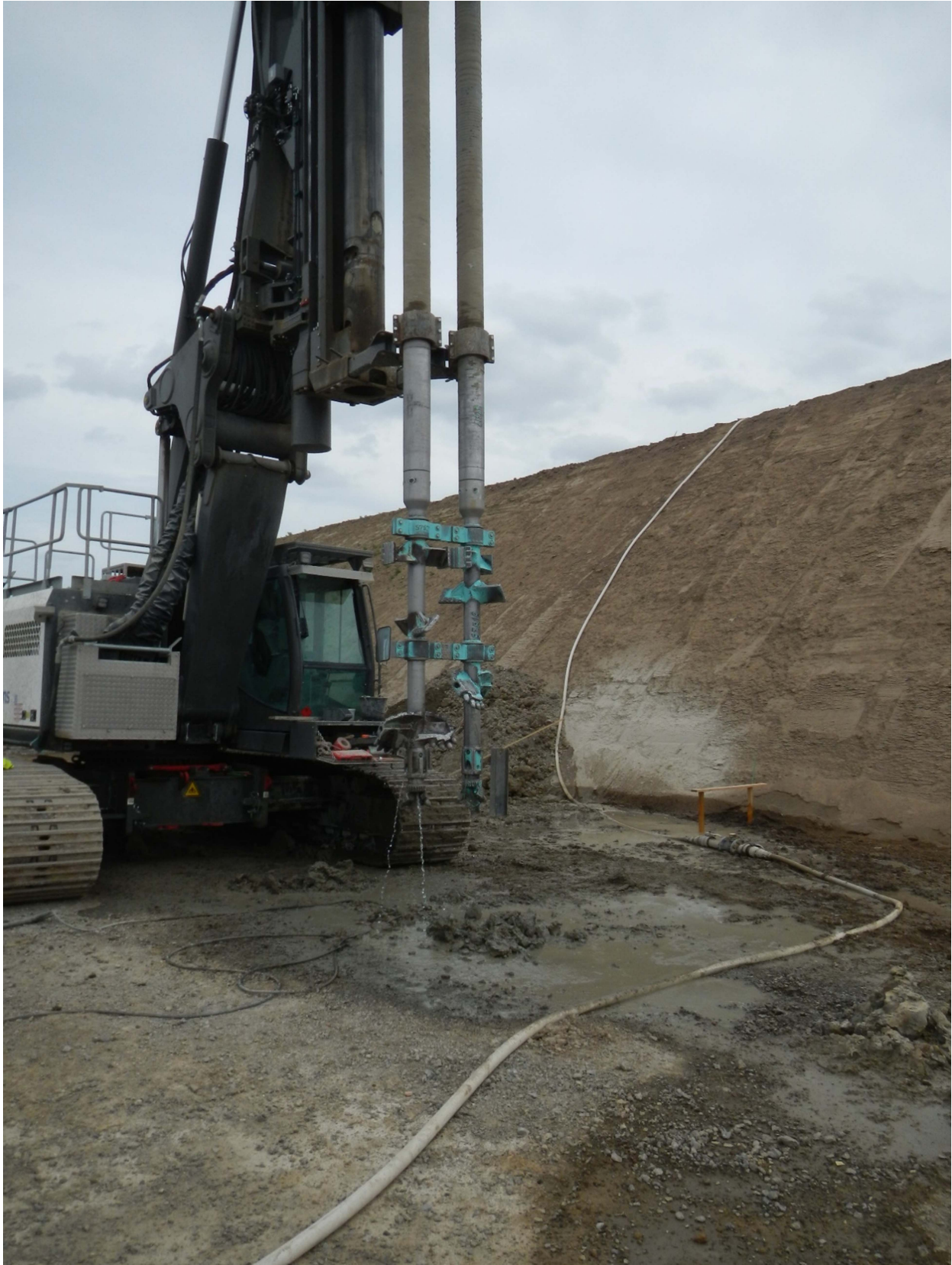
Fig. 11. Execution of secant soil-cement columns in double shaft configuration with two ABI drilling/mixing heads (with the courtesy of Franki Foundations – group Besix)
