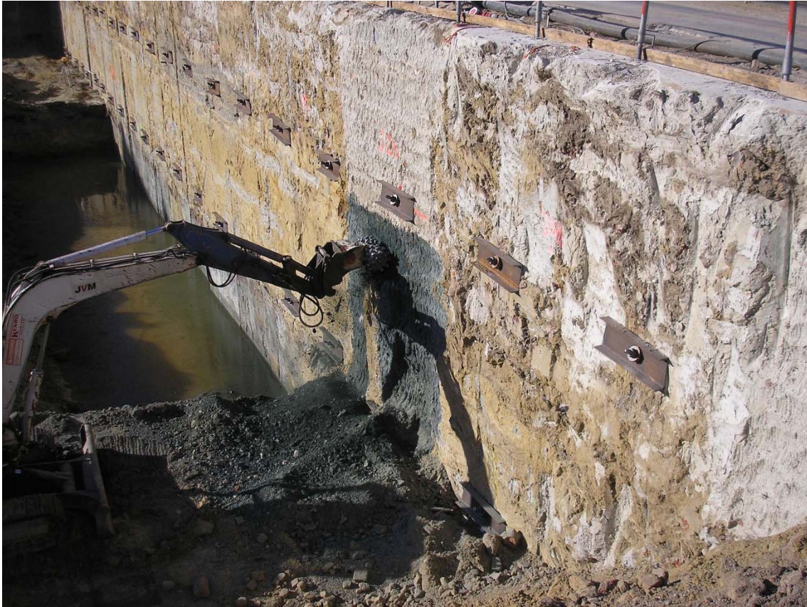
Fig. 22. Milling of the surface of the soil mix material of a soil mix wall made of CSM panels
