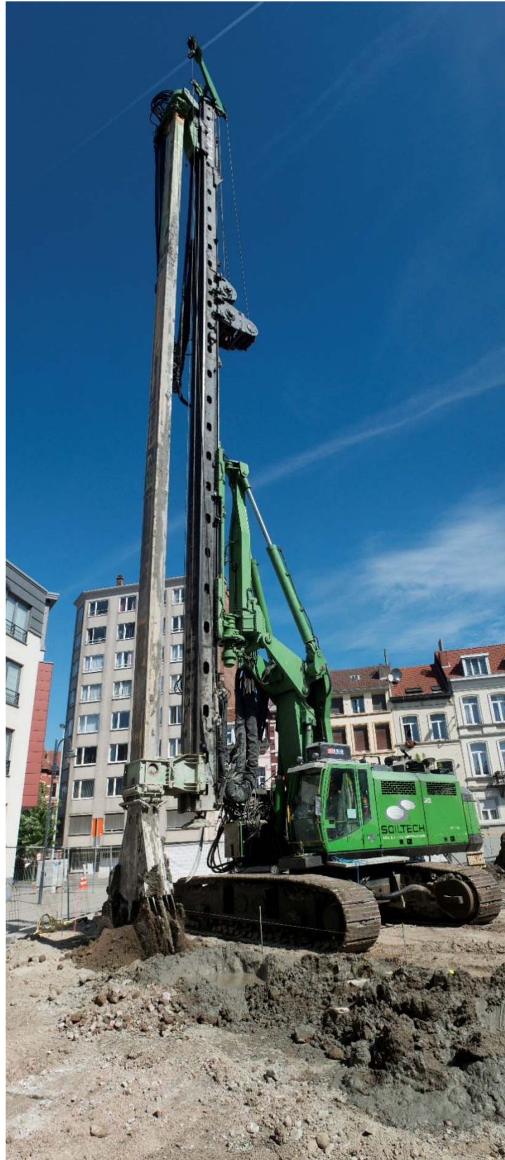
Fig. 15. Execution of a soil mix wall with secant panels performed with the CSM – the cutters are mounted on a square section kelly (with the courtesy of Soetaert nv – group Jan De Nul)
