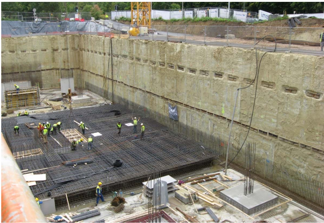
Fig. 4. Anchored soil mix wall (made with the CSM technique) used as retaining structure for the realization of an excavation (with the courtesy of Lameire funderingstechnieken nv)
