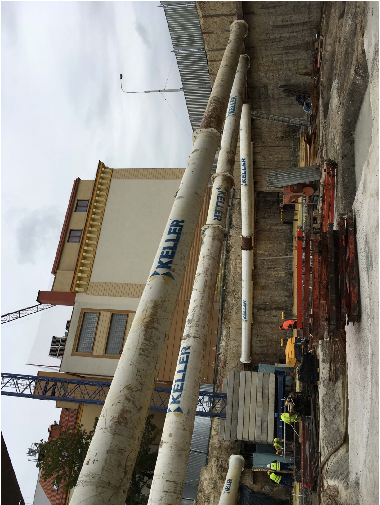
Fig. 2. Braced soil mix wall (made with soil-cement columns) used as retaining structure for the realization of an excavation, the bracing is performed after milling the soil mix surface (with the courtesy of Michał Topolnicki - Keller)
