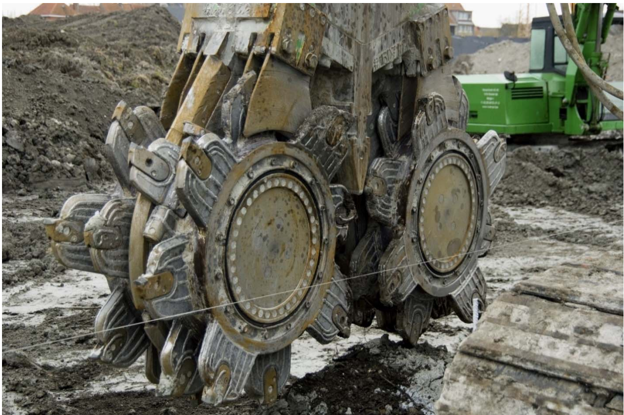
Fig. 16. Enlarged views of the cutter system of a CSM machine used for the execution of soil mix panels (with the courtesy of Soetaert nv – group Jan De Nul)
