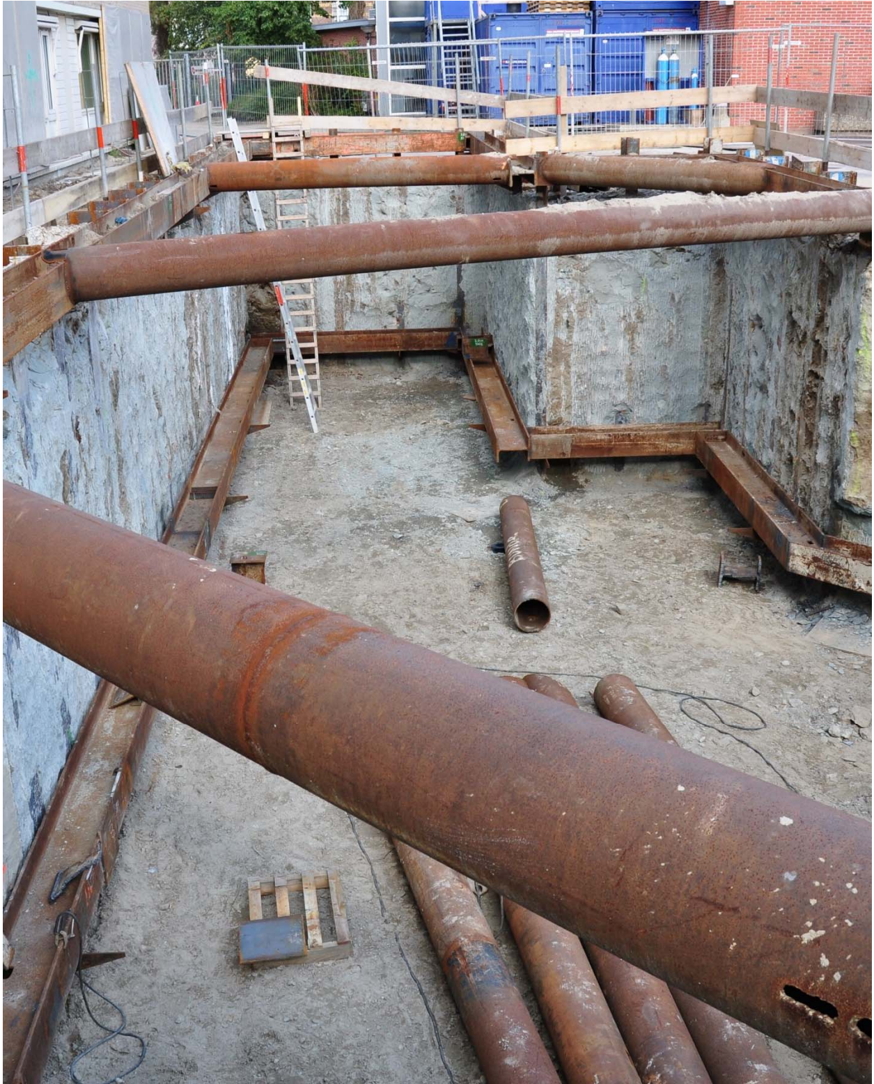
Fig. 1. Braced soil mix wall (made with the CSM technique) used as retaining structure for the realization of an excavation (with the courtesy of Bauer Nederland)
