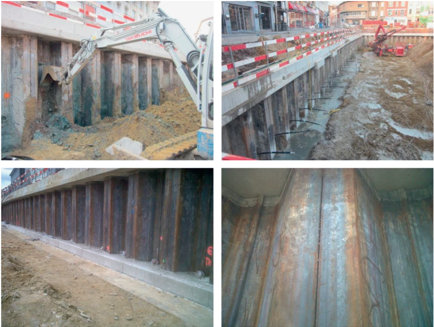
Figure 11.25 Progressive excavation and anchoring of the composite retaining wall. (Source: After Leemans (2012) ).
