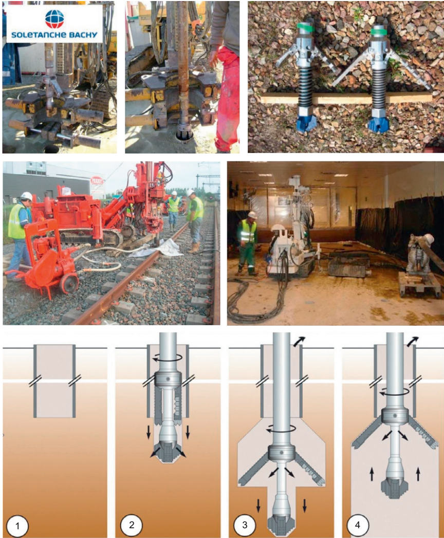
1. Casing installation 2. Introduction of the tool 3. Spreading of the tool and soil mixing 4. Withdrawal of the tool
