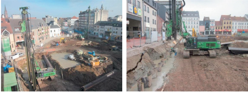
Figure 11.24 Installation of the sheet piles into the fresh soil mix material. (Source: After Leemans (2012) ).
